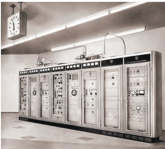
1963: VHF radio transmitter with 2 × 5 kW
